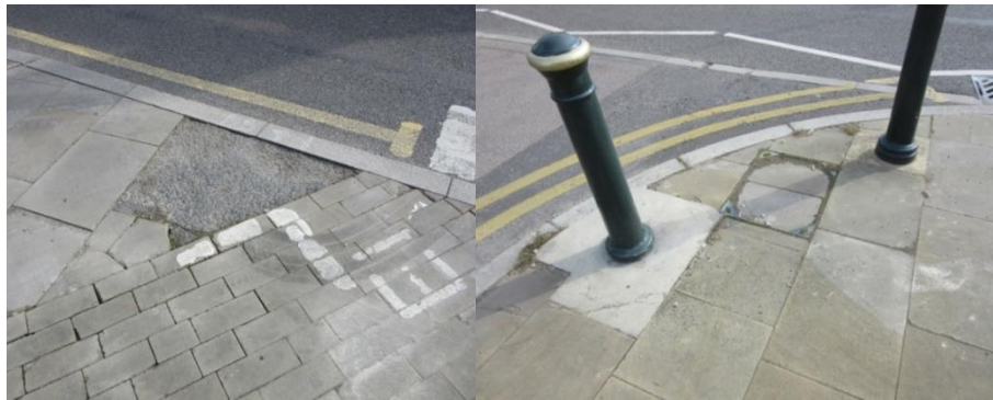
Figure 6.4. Examples in Wheathampstead High Street of poor repairs following works involving the pavement
